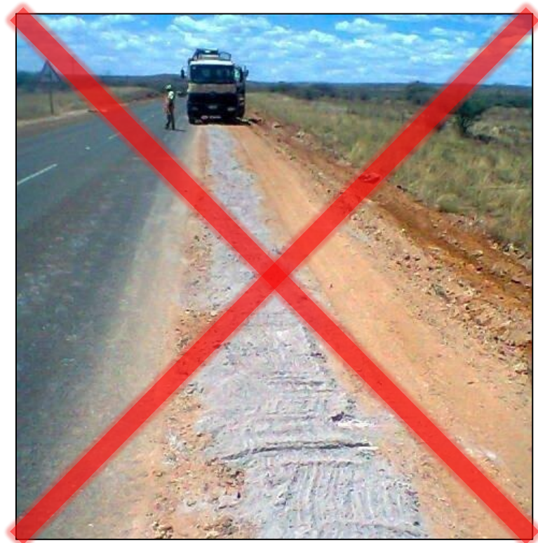
Figure 74. Example of Incorrect Spreading of Cement Prior to Stabilization
