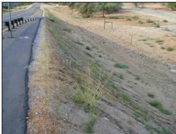
Figure 71. Side Slope Erosion due to Inadequate Compaction
