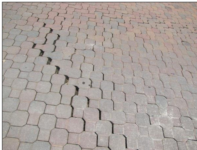
Figure 107. Excessive Openings in an Area Paved with Type S-C Blocks
