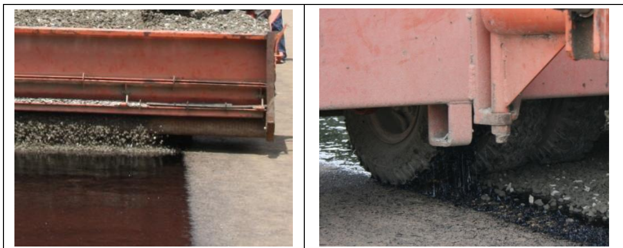
Figure 90. Binder Not Fully Covered by Aggregate
