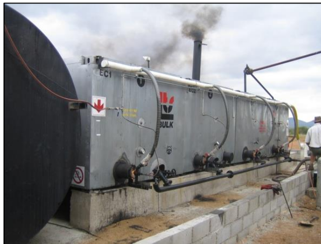
Figure 20. Bitumen Binder Storage Tanks
