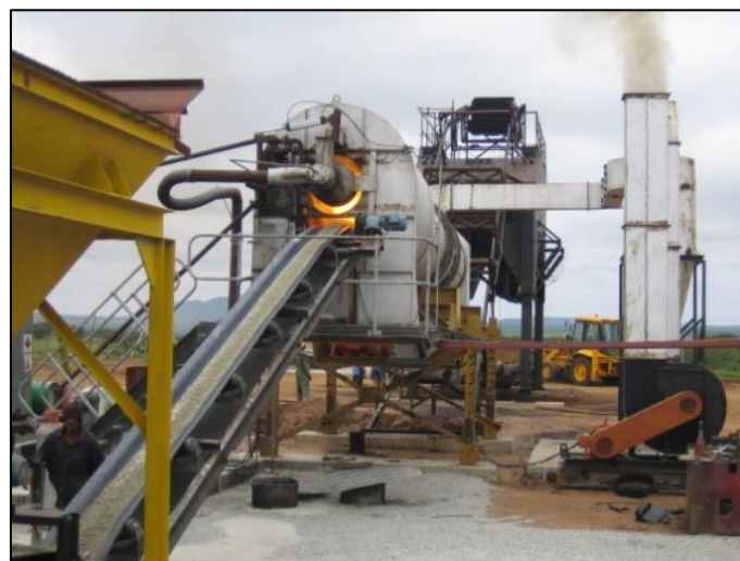
Figure 19. Cold Feed Bins with Conveyor
