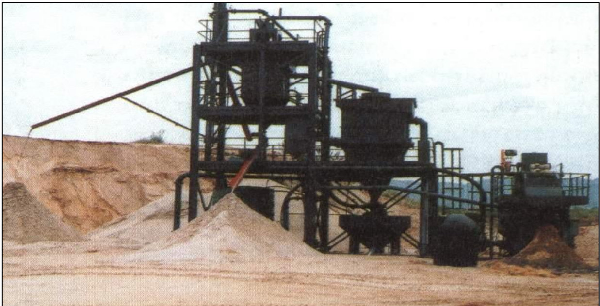
Figure 7. Cyclone Crusher Plant
