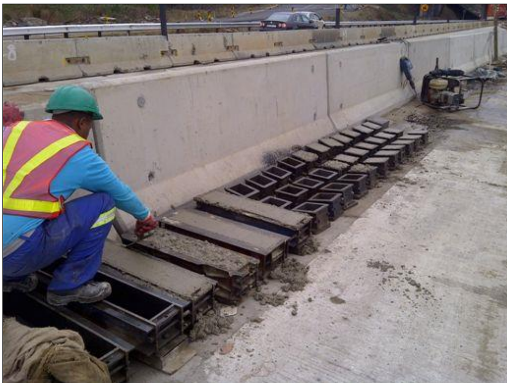
Figure 23. Inappropriate Site Manufacture of Concrete Specimens
