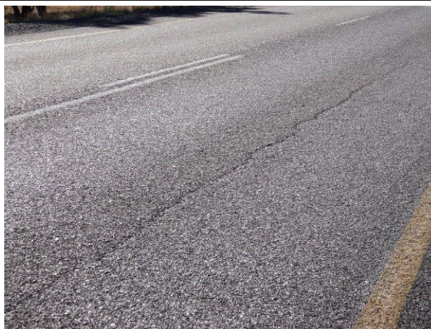
Tree Causing Crack
