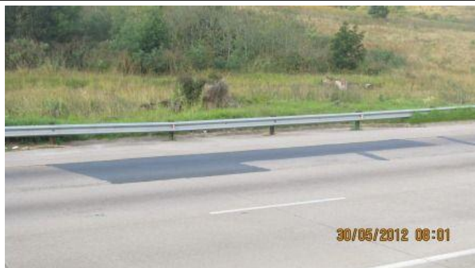
Tree (showing as stump) Causing Distress Resulting in Extensive Patching
