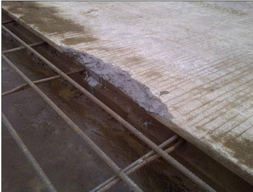
Figure 22. Spalled Edge from Side Form Removal
