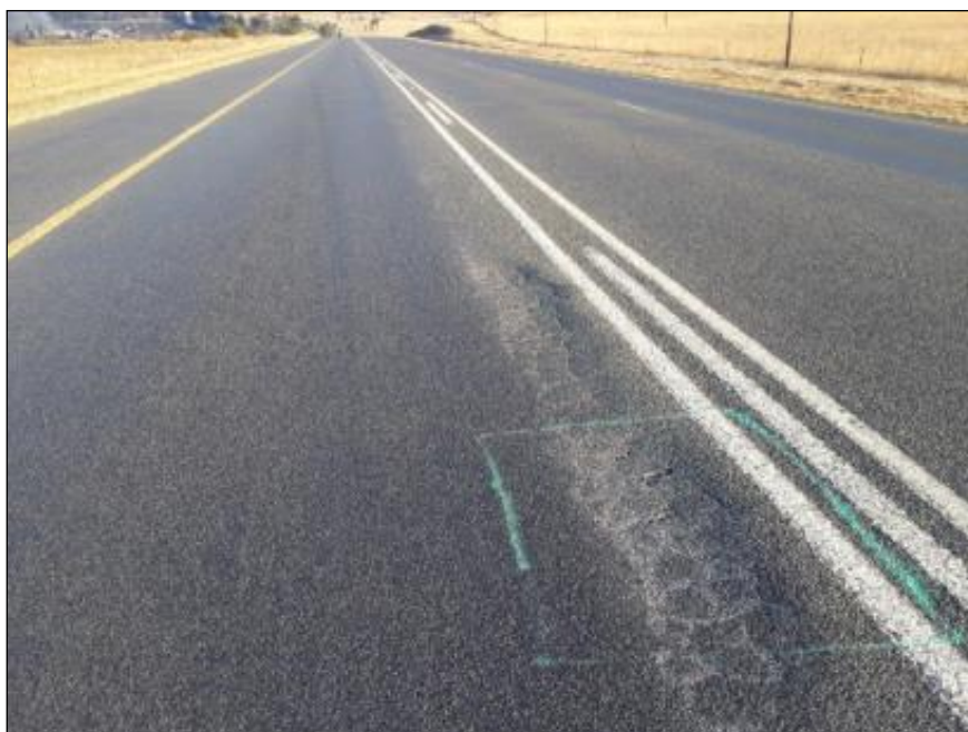
Figure 5. Typical Failure Along a Poorly Constructed Longitudinal Construction Joint of a G1 Base Layer
