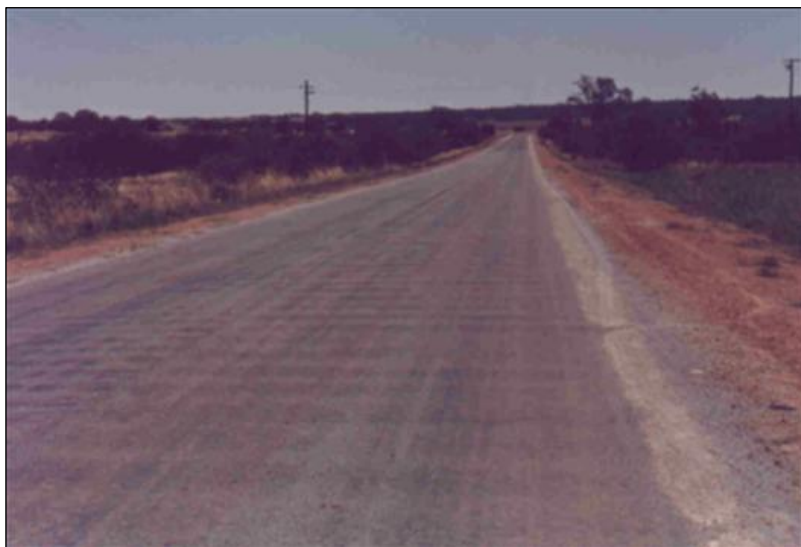
Figure 18. Empty Chip Spreader causing Corrugations
