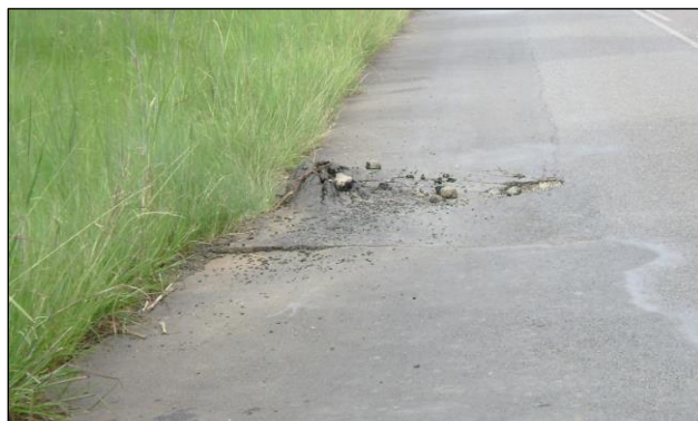
Figure 7. Moisture Accelerated Distress
