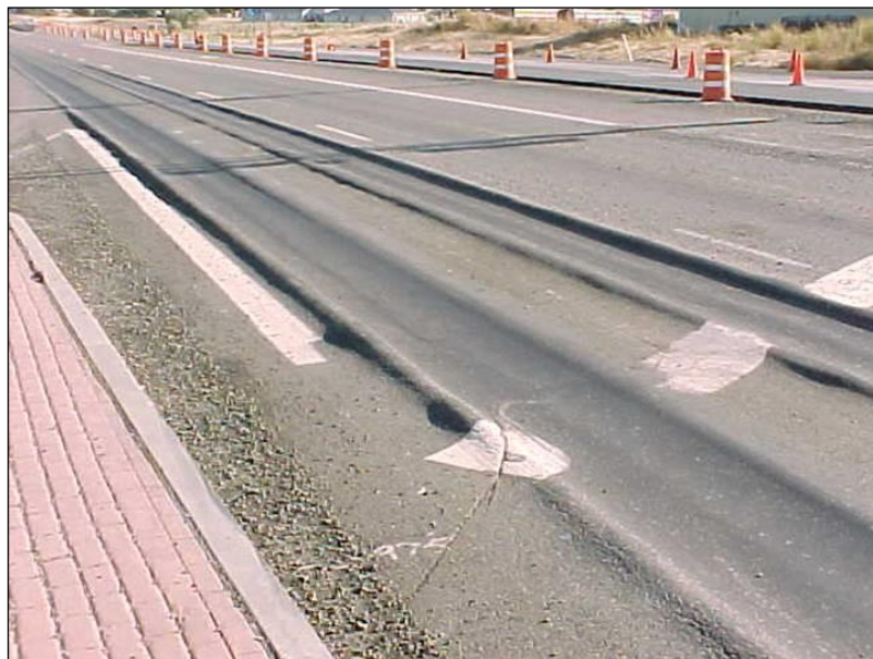
Figure 32. Narrow Wheelpath Rutting
