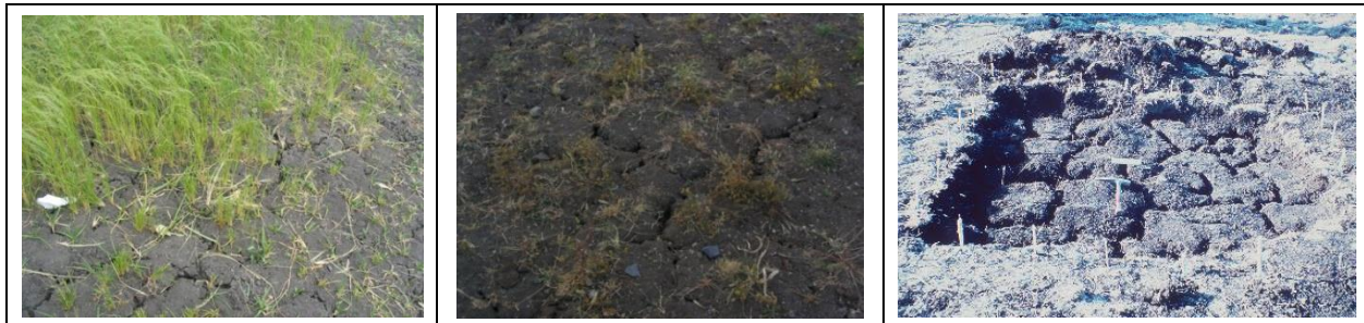
Figure 15. Examples of Shrinkage Cracking
