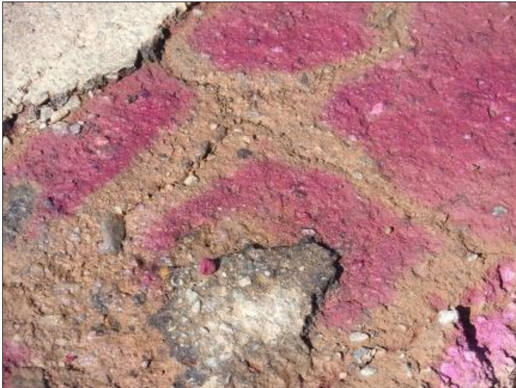
Figure 44. Effect of Carbonation Adjacent to Cracks in a Stabilized Layer
