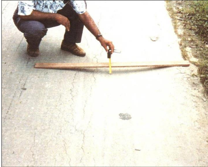
Figure 31. Wide Subgrade Rutting
