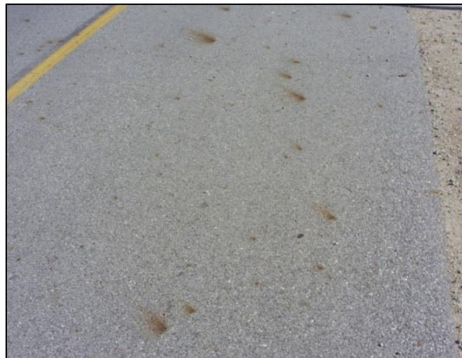
Figure 20. Asphalt Staining from Oxidation of Sulphides
