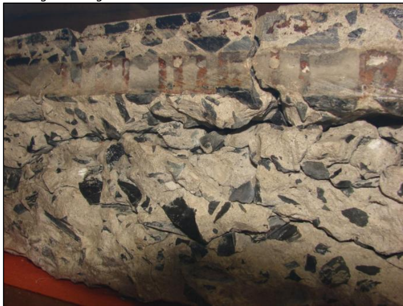
Figure 19. Concrete Failure due to Alkali-Silica Reaction
